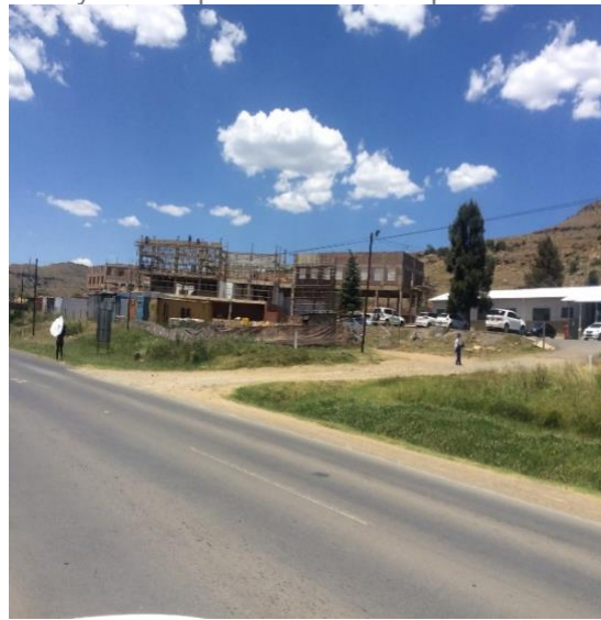
Delayed completion of municipal offices
