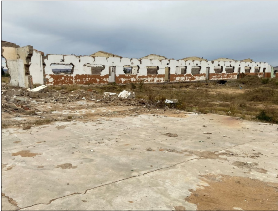
Figure 7: The dilapidated building of a local school. Photograph by Nonkululeko Zondo
